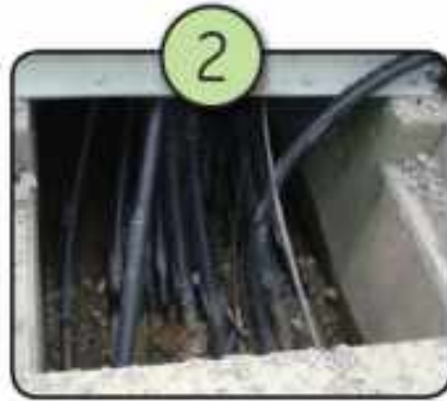
Traditional cable trenches
