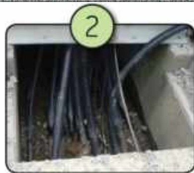
Traditional Cable Trench
