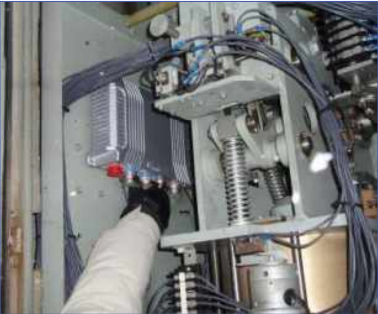
Internal, old oil-type Circuit Breaker
