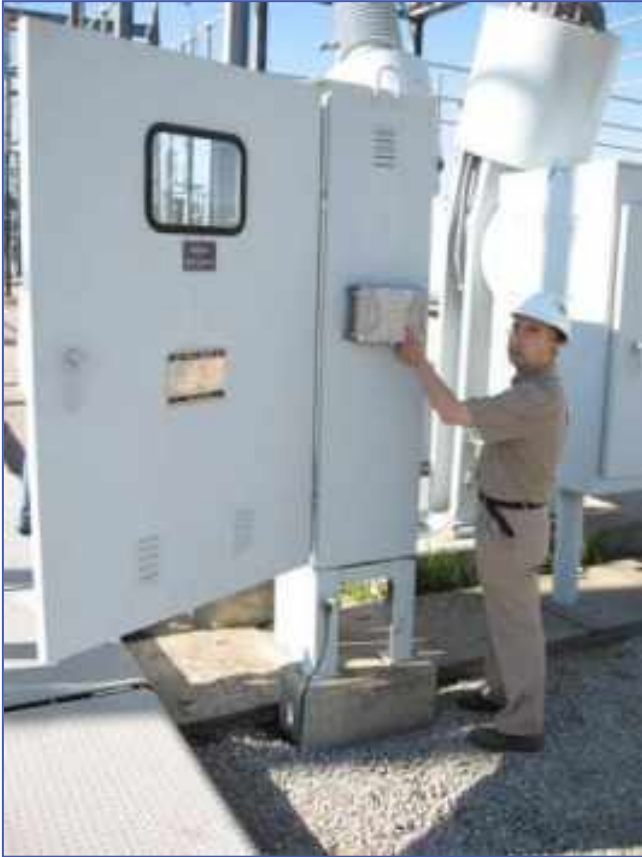
External, on a Circuit Breaker
