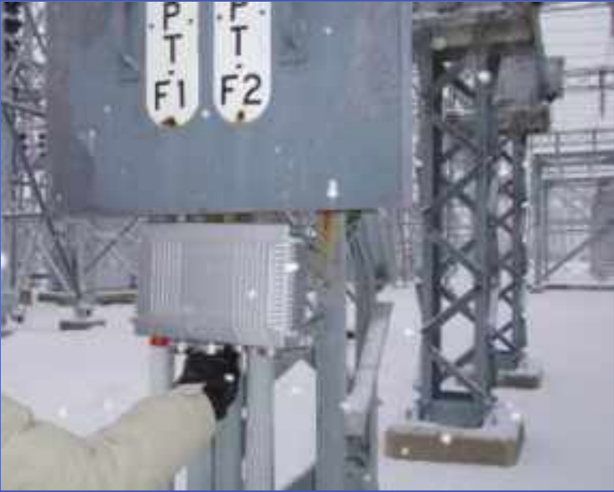
External, below VT marshalling box
