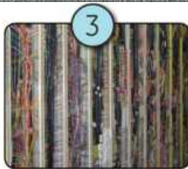
Thousands of Copper Wires from Switchyard
